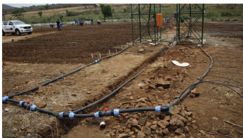
System operability check completed with excellence, 2023
